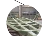
The hull is reinforced with a longitudinal and transverse floor grid system including stringers which also supports the keel fittings, bulk heads, keel stepped mast, engine frame, tanks, and cabin soles. The grid system is in the same material and E-module as the hull. Made in sandwich construction with vinylester on both inner and outer skin and Divinycell as core. It is glued and laminated to the hull. The whole structure is super strong and weighs about 900 kg.
