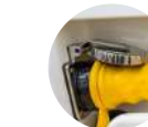
230V shore power system fitted with stainless steel intake, 50 m cable, fuse box, earth fault interruptor and four sockets.
